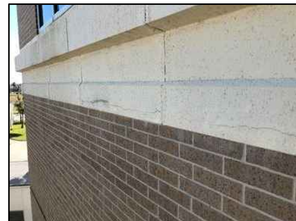
CRACKS IN THE EIFS TRIM
