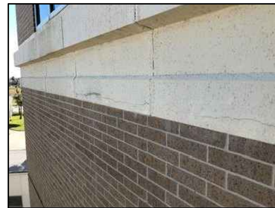
CRACKS IN THE EIFS TRIM
